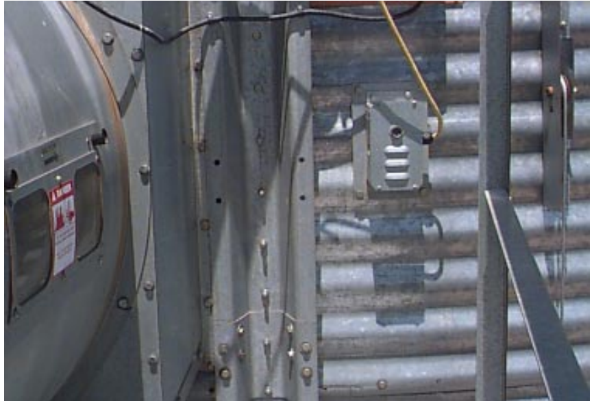
Airswitch mounted on the bin sidewall.
